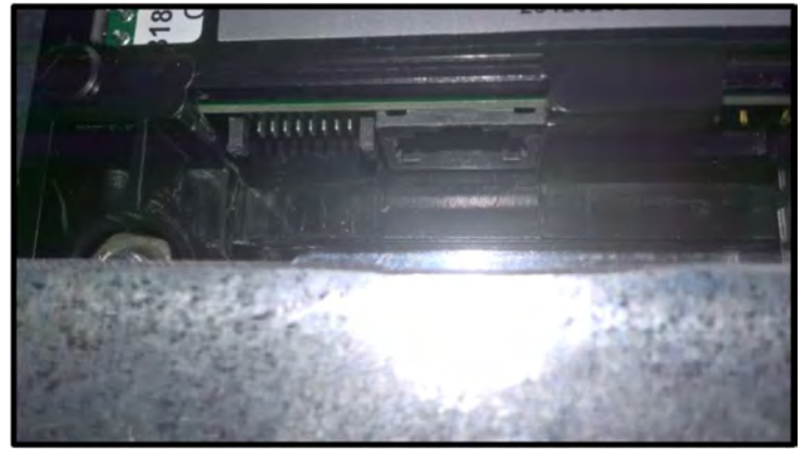
Slot for connection of loose ethernet cable.
